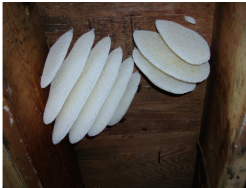
New wax combs between basement joists
